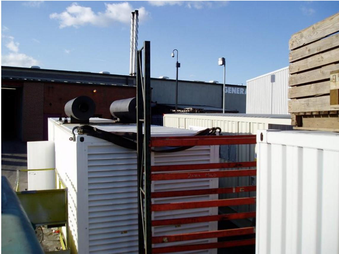
Figure 6.4: Example generator enclosure with high specification exhaust silencers
