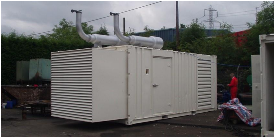
Figure 6.2: Mud pump engine enclosure (note exhaust silencers)
